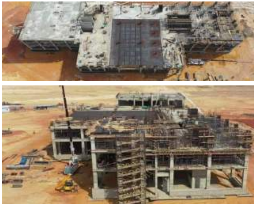
Figure 2-6 Photos from the Mohamed Naguib station ( regional station type )
