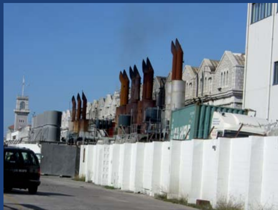
OESCO Power Station
