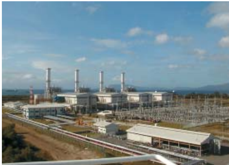
100 km south of Manila, the largest and the most modern power plant of the Philippines is under construction. Siemens AG is constructing the second gas and steam turbine power plant San Lorenzo (500 MW) as a turn key plant near by the 1,000 MW power plant Santa Rita (see picture above). This is a BOT-type project. Within the frame of project and export financing, the KfW grants credits as well as investment loans (in order to finance the local costs).
