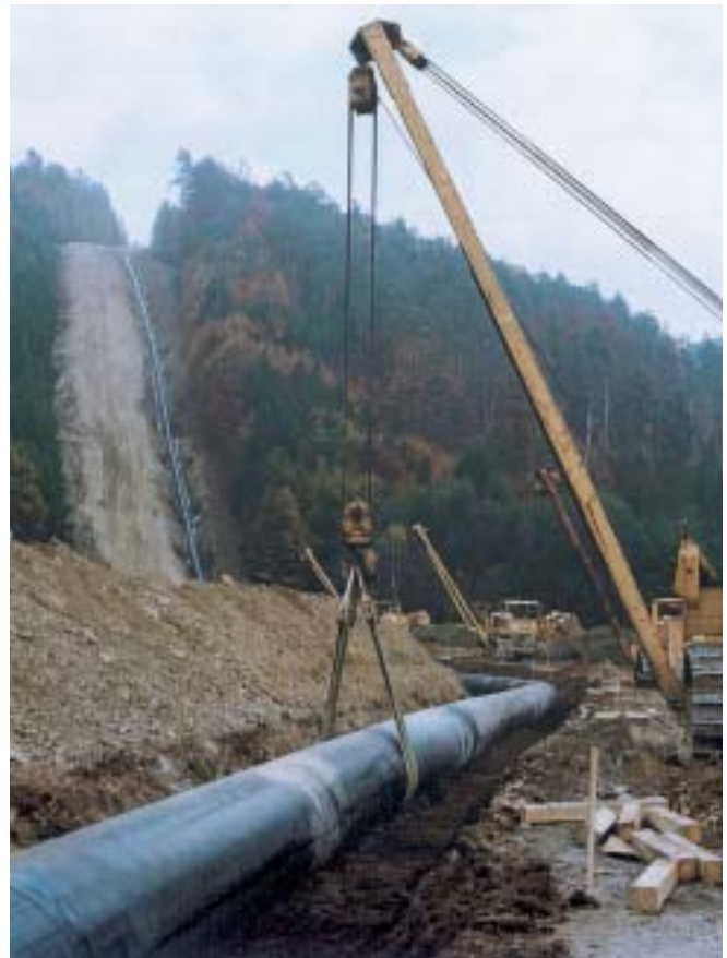
The production of large pipes by a joint venture in St. Petersburg between Europipe GmbH (Mannesmannröhrenwerke /Dillinger Hüttenwerke) and the Russian steel group Severstal is to improve the supply of the country with gas and oil pipelines.
